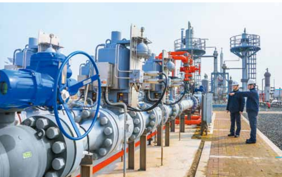
Our underground natural gas storage facility in Jintan, Jiangsu province, will facilitate the management of our gas inventory in East China during high-demand periods.
